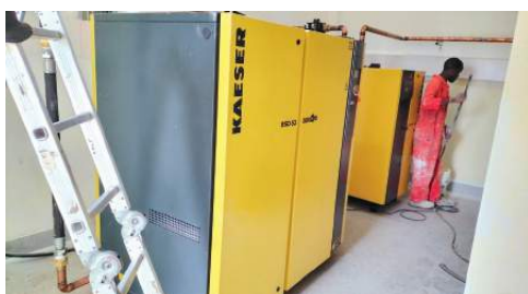
Medical Air System 2350L/ Min Duplex Configuration Medical Air Plant Installed, Tested And Commissioned.
