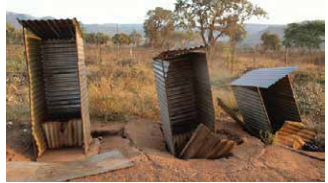
Dilapidated pit latrines in a learning institution
